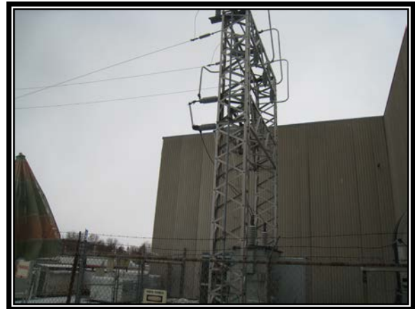
Transformer (West Elevation)
